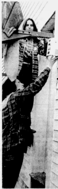
Job Site Supervisor Susan Shaw (left) observes Youth Experience workers Babs Deslauriers (top right) and Mary McDonald painting the exterior of the Thompson Town Hall, as part of a renovation project begun April 1.
